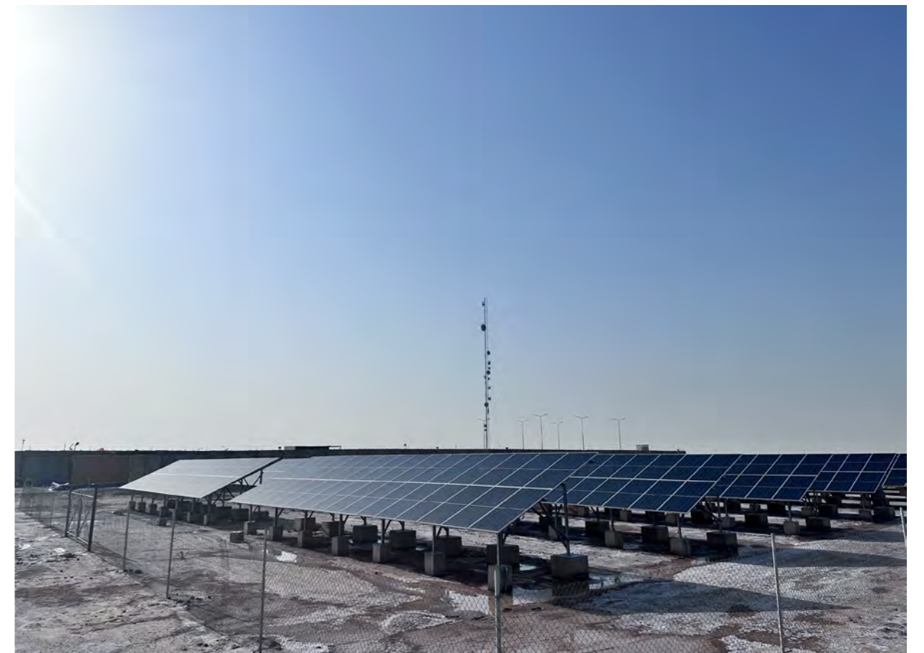
KEBL Camp Oilfield Photovoltaic Power Station Project
