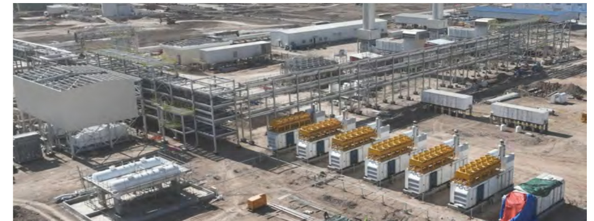
Rental Power Plant in KEBL
